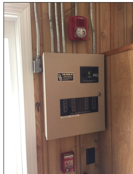
Existing Fire Alarm Control Panel
