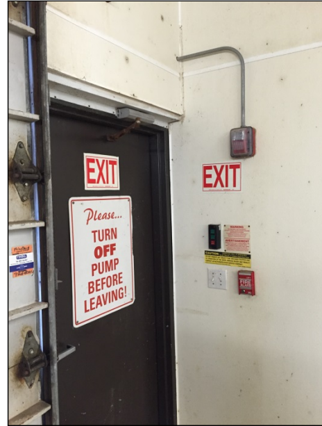
Plastic Non-Illuminated Exit Sign
