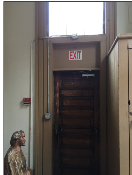
Plastic Non-illuminated Exit Sign
