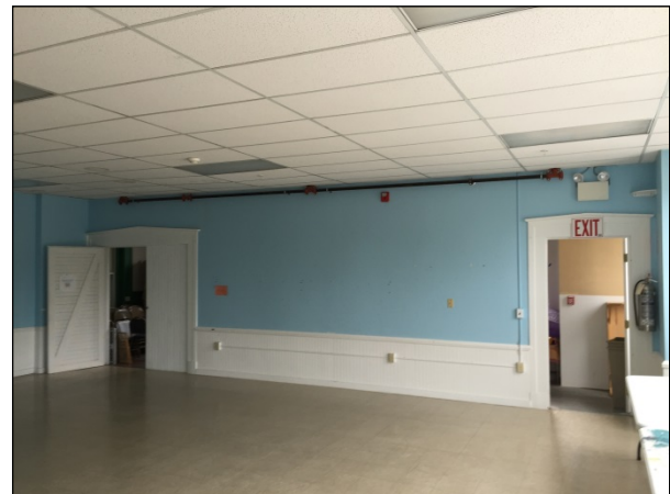
Exit Sign and Remote Battery Unit Heads
