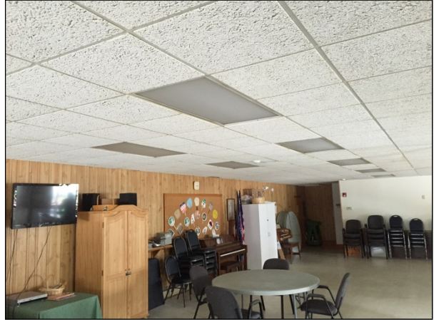
Recessed Mounted Fluorescent Fixtures
