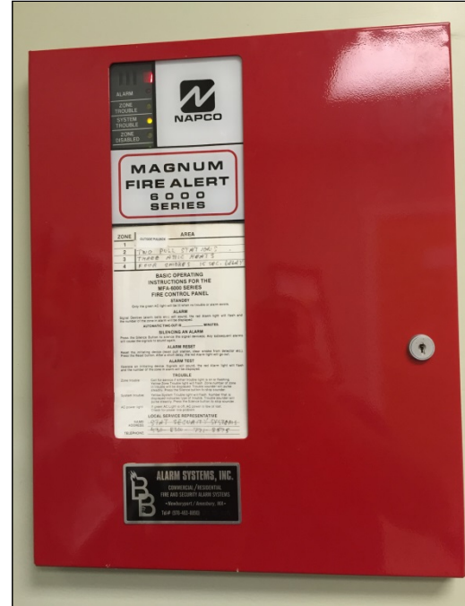
Fire Alarm Control Panel
