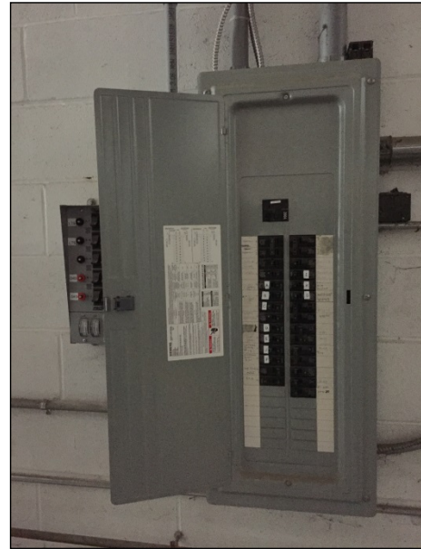
Main Electrical Service Panelboard
