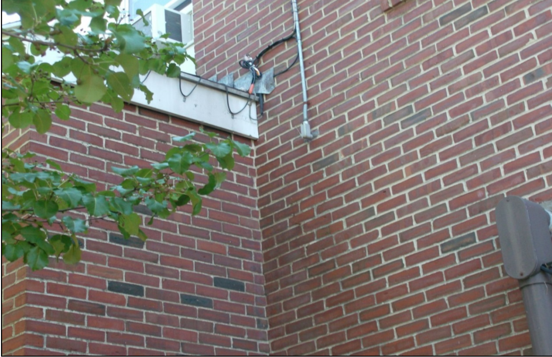
Valley over main entrance. Ice dams are a constant problem, note heat tape.
