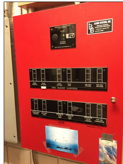
Existing Fire Alarm Control Panel
