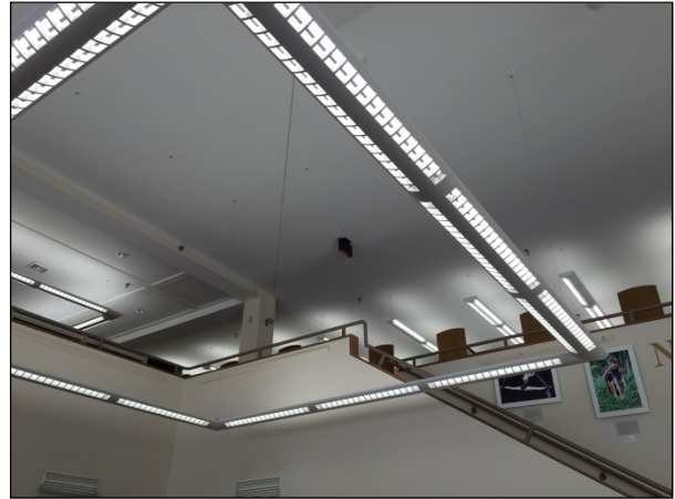
Pendant Mounted Fluorescent Fixtures
