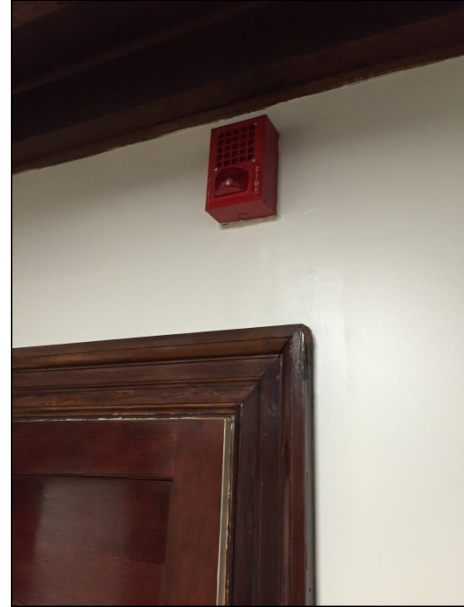
Existing Fire Alarm Audio Visual Device
