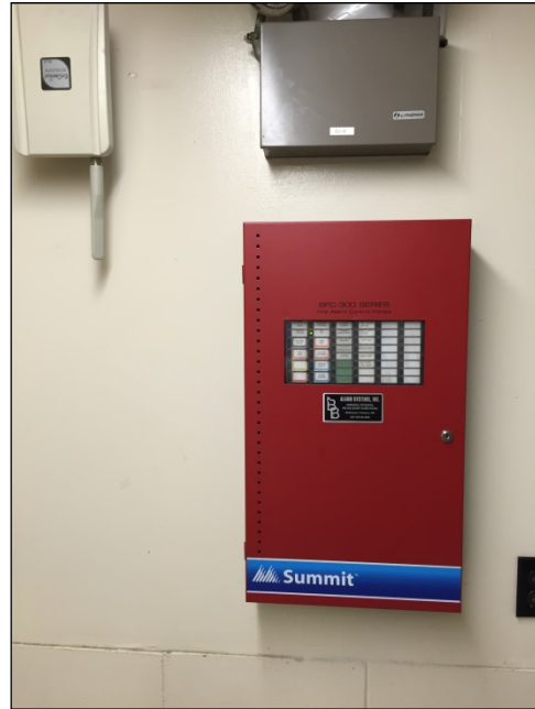
Existing Fire Alarm Control Panel
