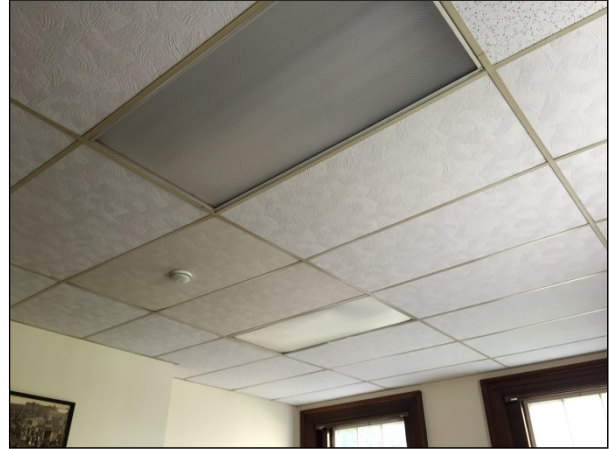
Recessed Mounted Fluorescent Fixtures
