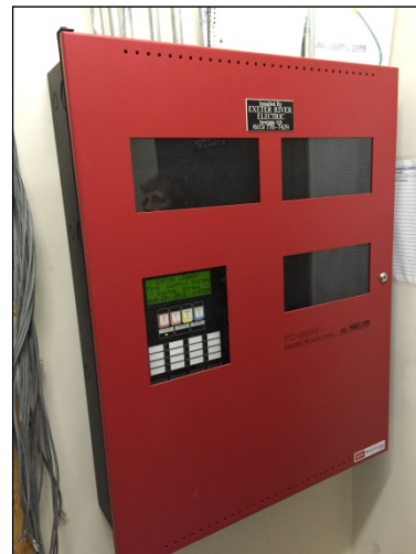
Existing Fire Alarm Control Panel
