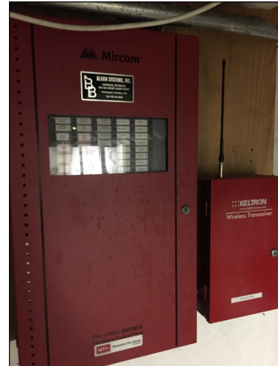
Existing Fire Alarm Control Panel
