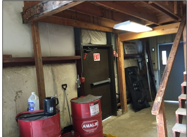
Plastic Non-Illuminated Exit Sign
