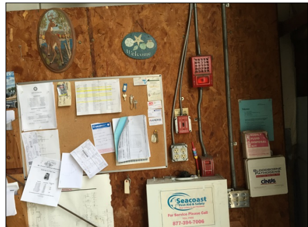
Pull Station with NON-ADA Type
