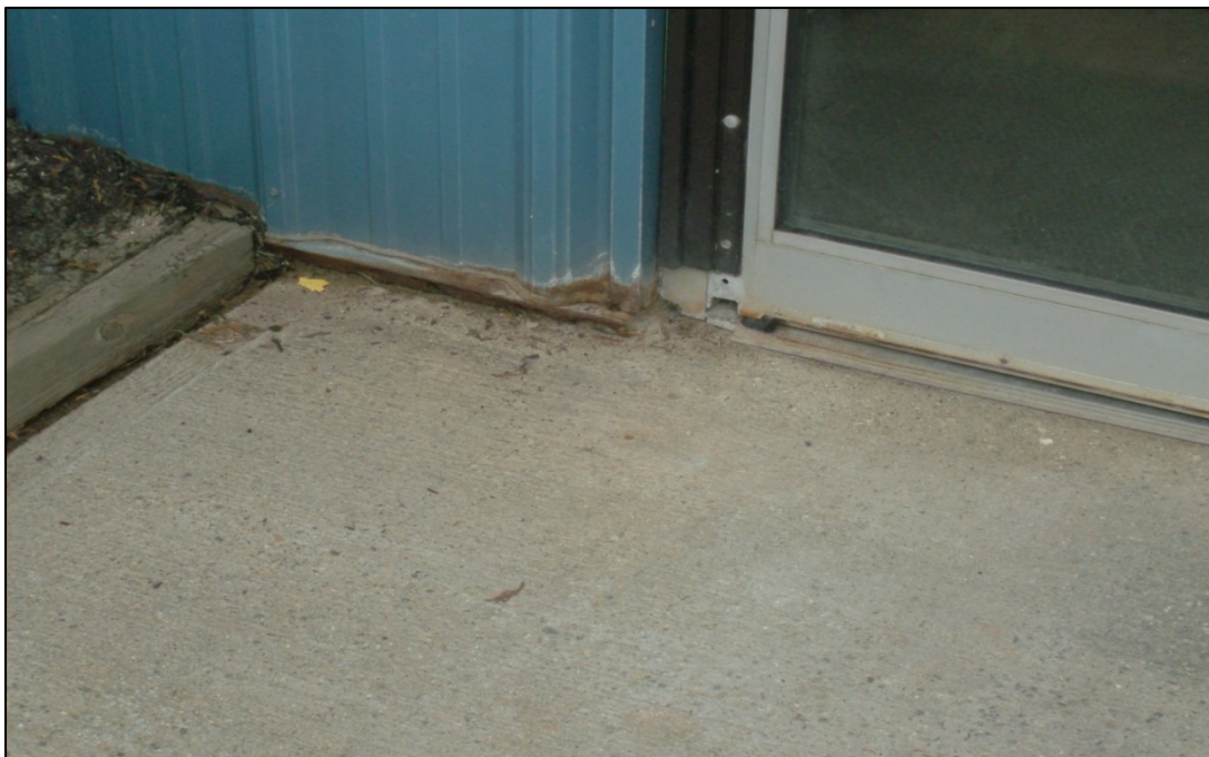
Corrosion at bottom of door and siding at entrance to offices.
