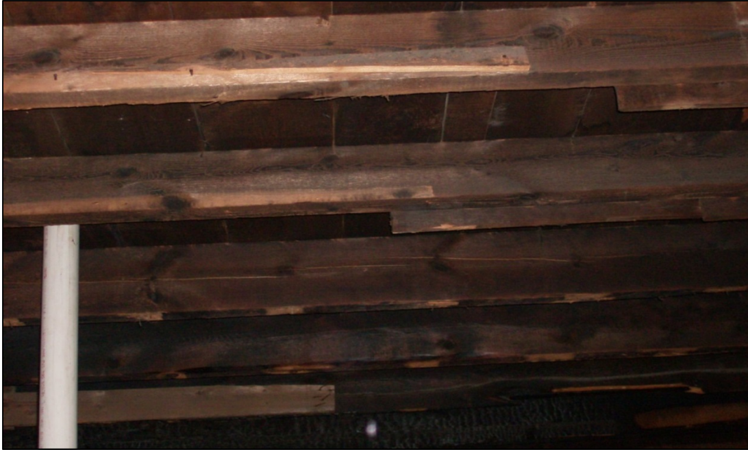
Former second floor ceiling framing members with slight charring.
