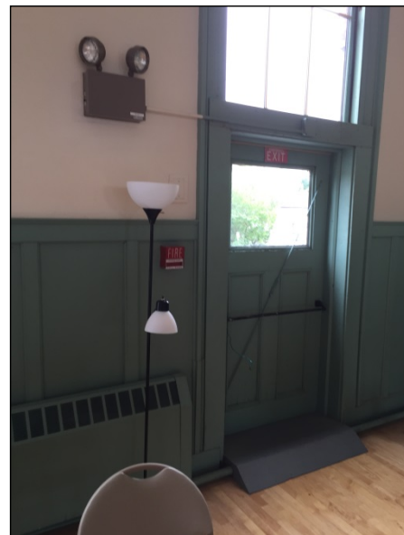
Existing Fire Alarm Pull Station
