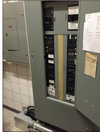
Main Electrical Service Panelboard
