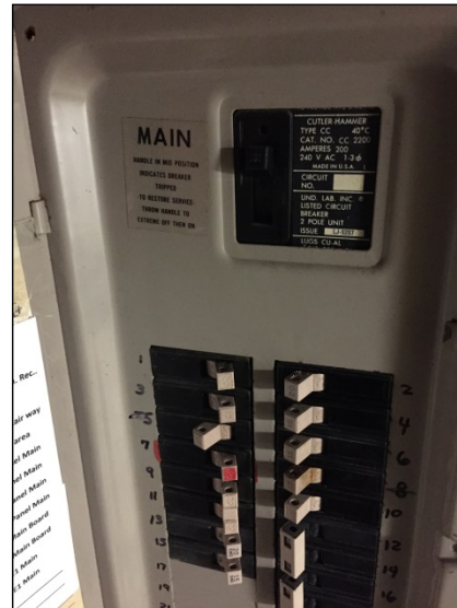
Main Electrical Service Panelboard
