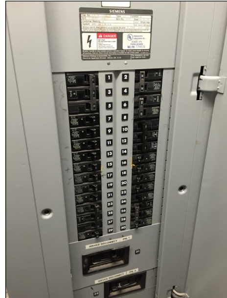
Main Electrical Service Panelboard
