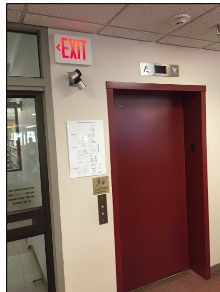
Exit Sign and Remote Battery Unit Heads
