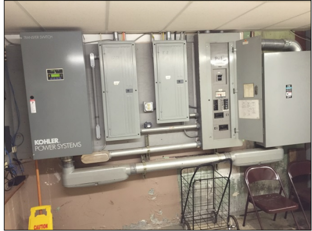
Main Electrical Service Lineup
