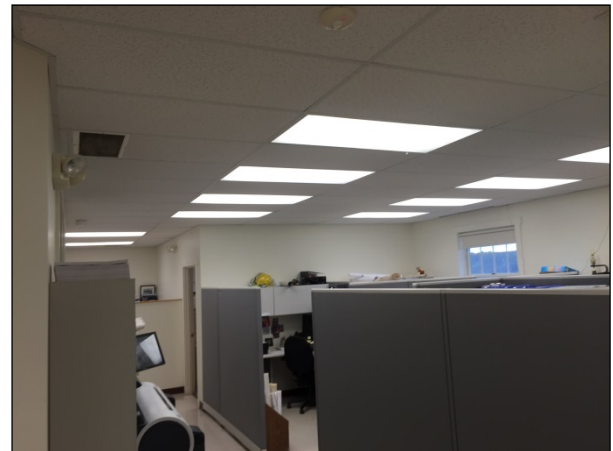
Recessed Fluorescent Lighting and Occupancy Sensor (ceiling mounted)
