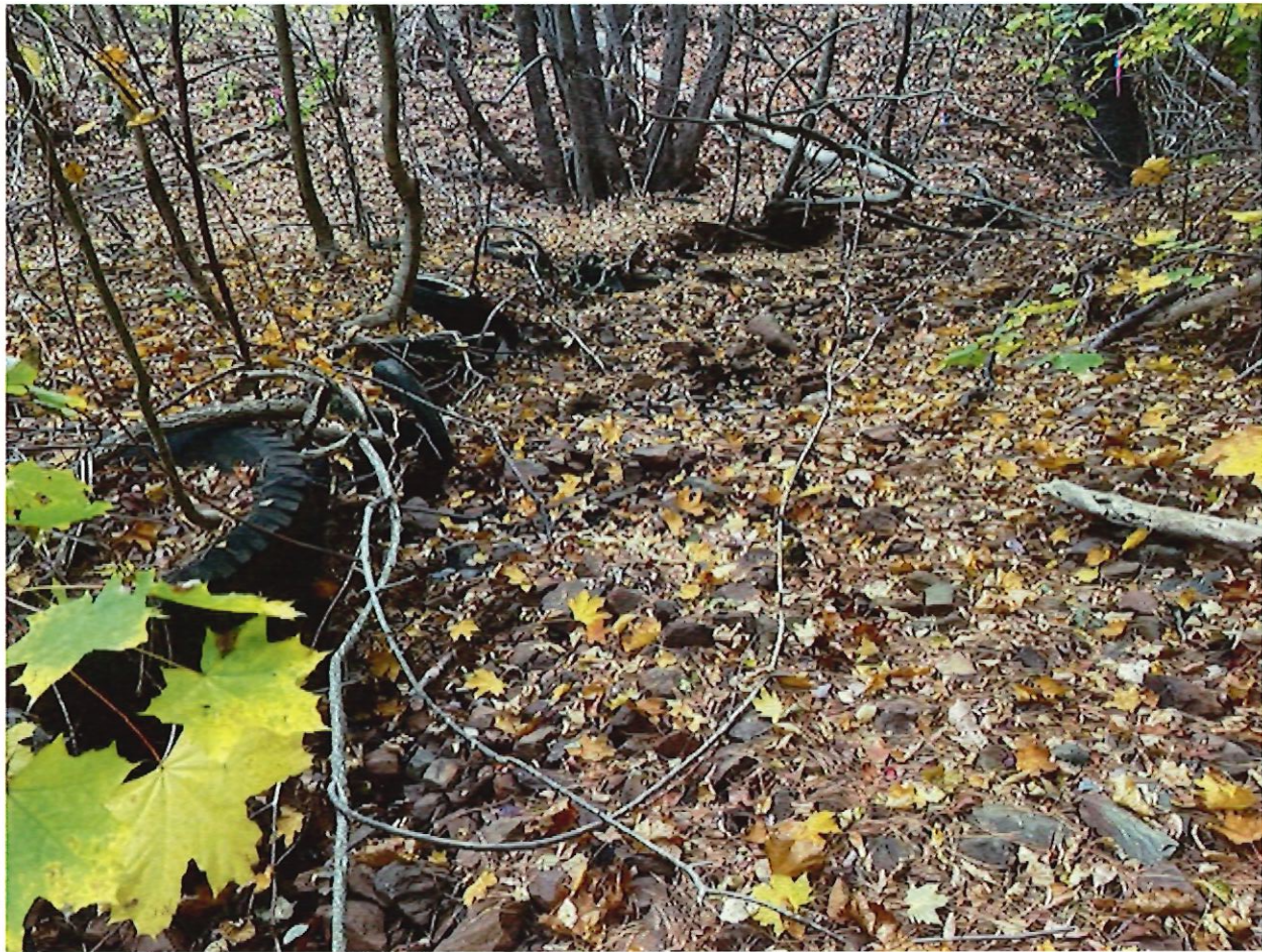
Rock-cobble bottomed stream – perennial flow. Man-made ditch, Note tires used to stabilize the slope.
