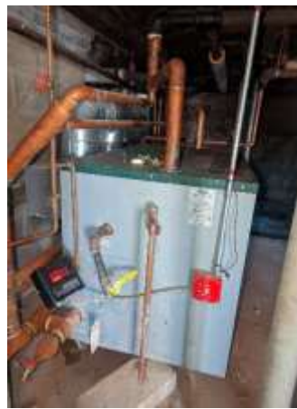
Figure 2: Existing Steam Boiler
