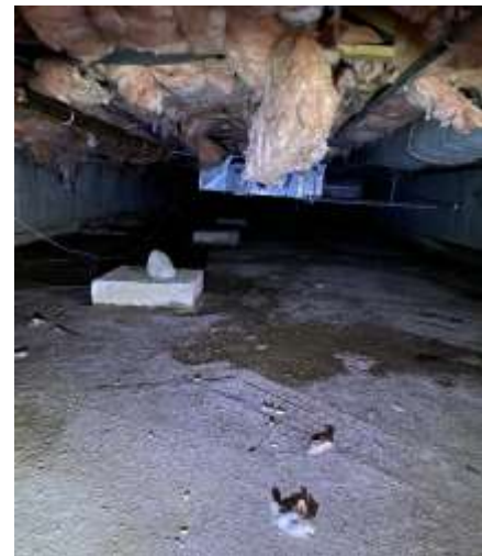
Figure 4: Failing FGB Insulation
