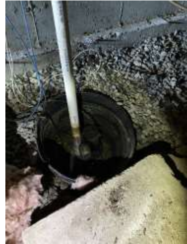
Figure 3: Existing Sump Pump
