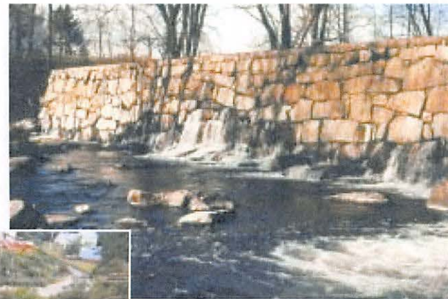
Below: Many dams in Maine are aging and in disrepair, such as the Collins Mill Dam on Cobbosseecontee Stream, West Gardiner.
