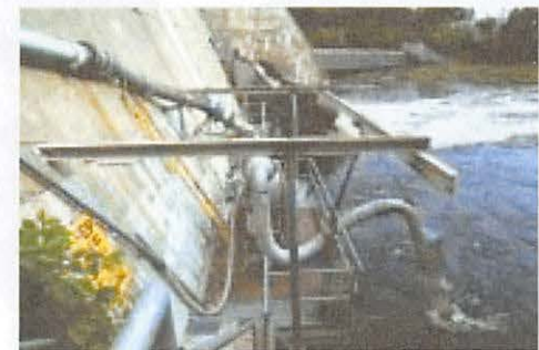
Fish pump at Ft. Halifax Dam on the Sebecook River.
