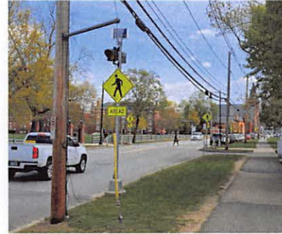
Advanced pedestrian crossing warning signs adjacent to Phillips Exeter Academy
